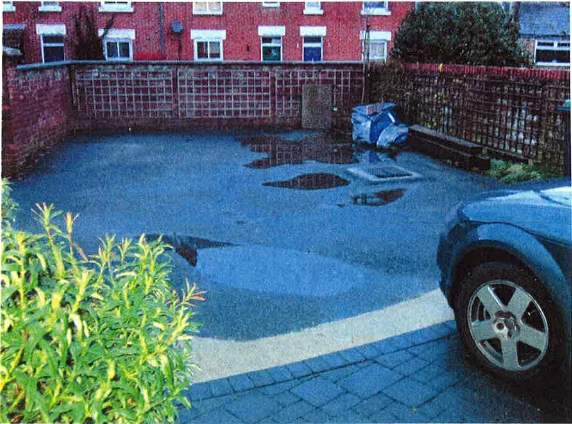
Puddles in Courtyard at No 78 Lower Rd.
